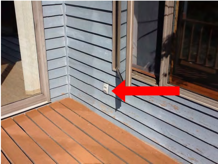
Exterior outlet is missing GFCI protection.
