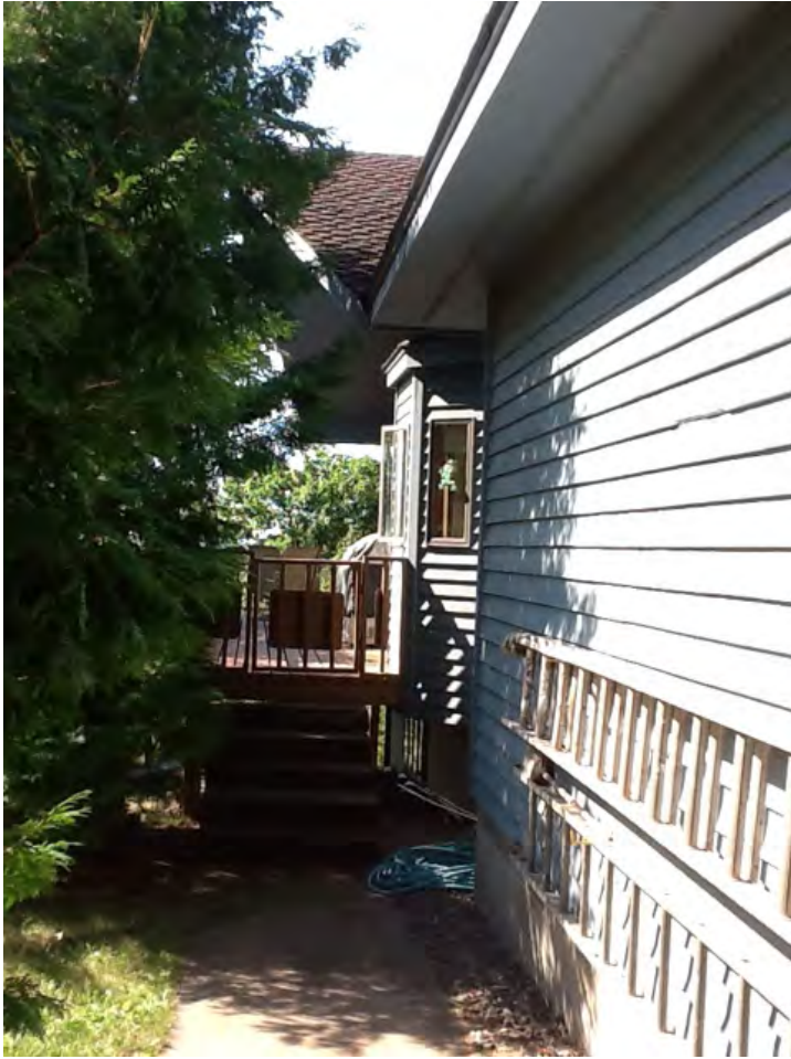
Recommend trimming back tree limbs from exterior to prevent excessive wear.
