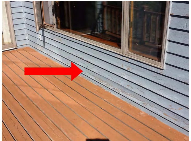
Recommend painting siding to extend useable life.
