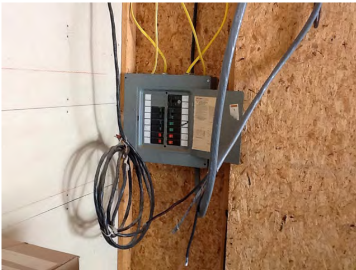
Sub-panel in garage. Wiring is not complete in this panel.
