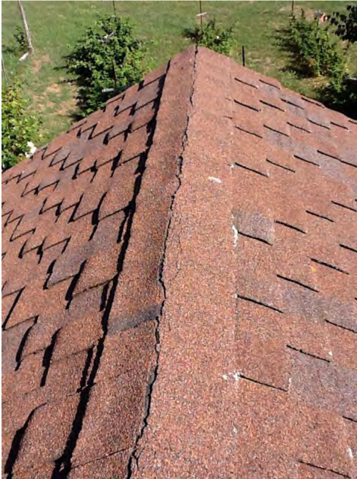
Ridge cap shingles are cracked.
