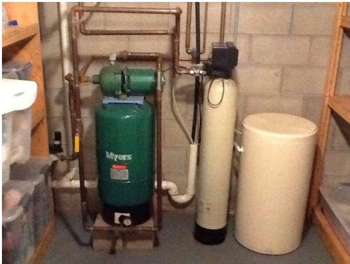
Well pressure tank, pump, and water softener system.
