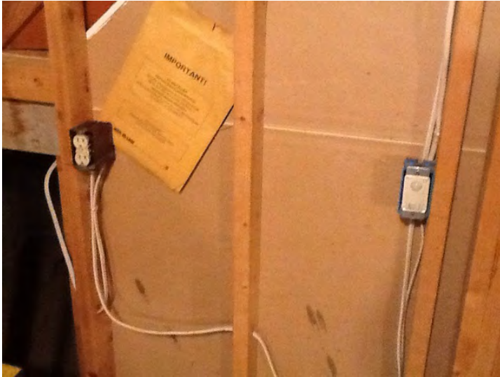
Missing coverplates present a safety hazard.
