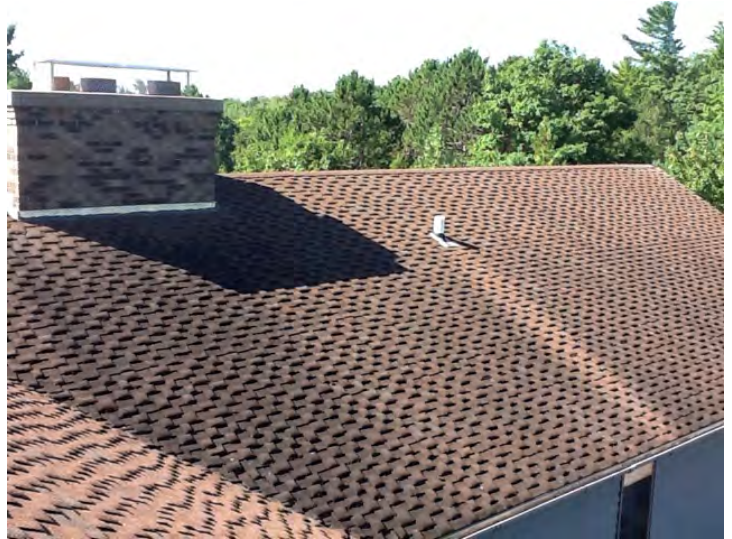
Asphalt architectural roof is showing normal signs of wear due to its age and is in marginal condition.
