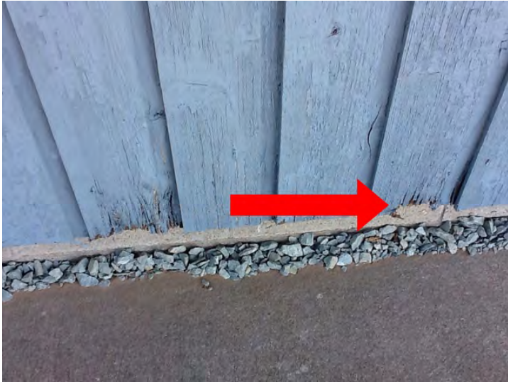
Visible wood decay along bottom courses of siding.
