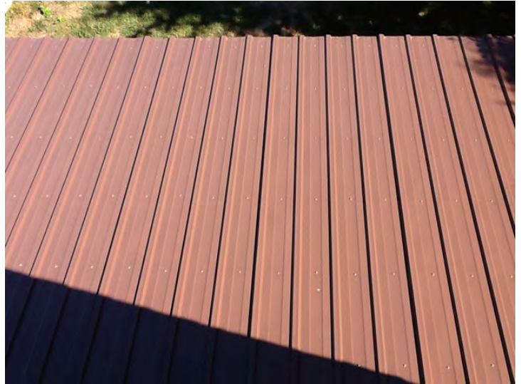
Metal roof over north garage addition was in satisfactory condition at the time of inspection.
