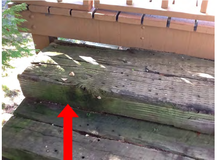
Loose railroad tie on top tread presents a safety hazard.
