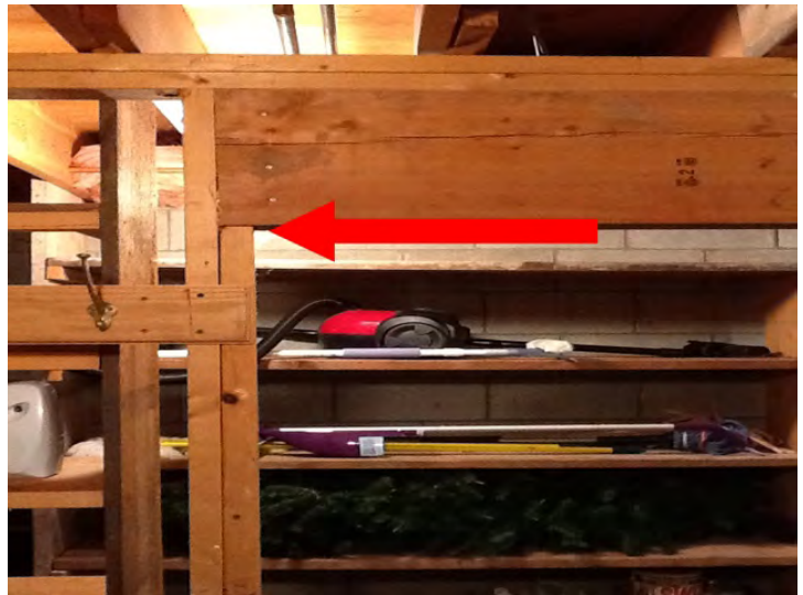
Recommend a bearing point of 3" on both sides of header beam in basement utility room.
