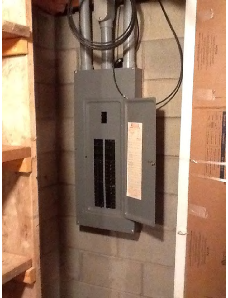
200 amp main electrical panel in basement utility room.
