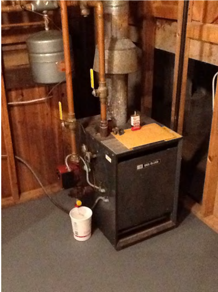
Weil-McLain boiler was in proper working order at time of inspection.
